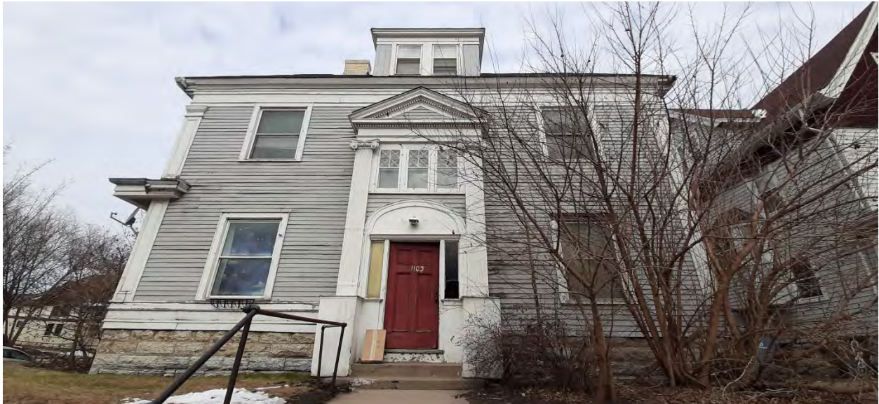
Front (south/southwest) elevation of 1103 4 th Street SE, From 4 th Street SE, looking north/northeast, November 2020, source: CPED
