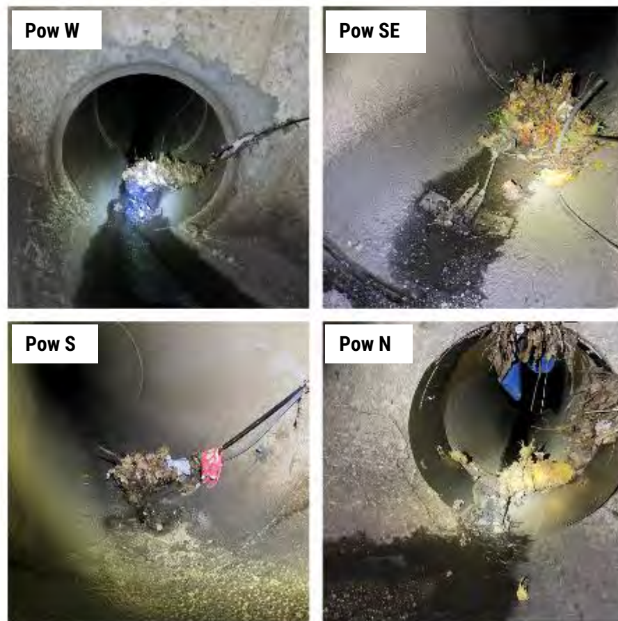
Figure 12. Photos of a disconnected intake tube and debris build up at each Powderhorn site in 2023.
