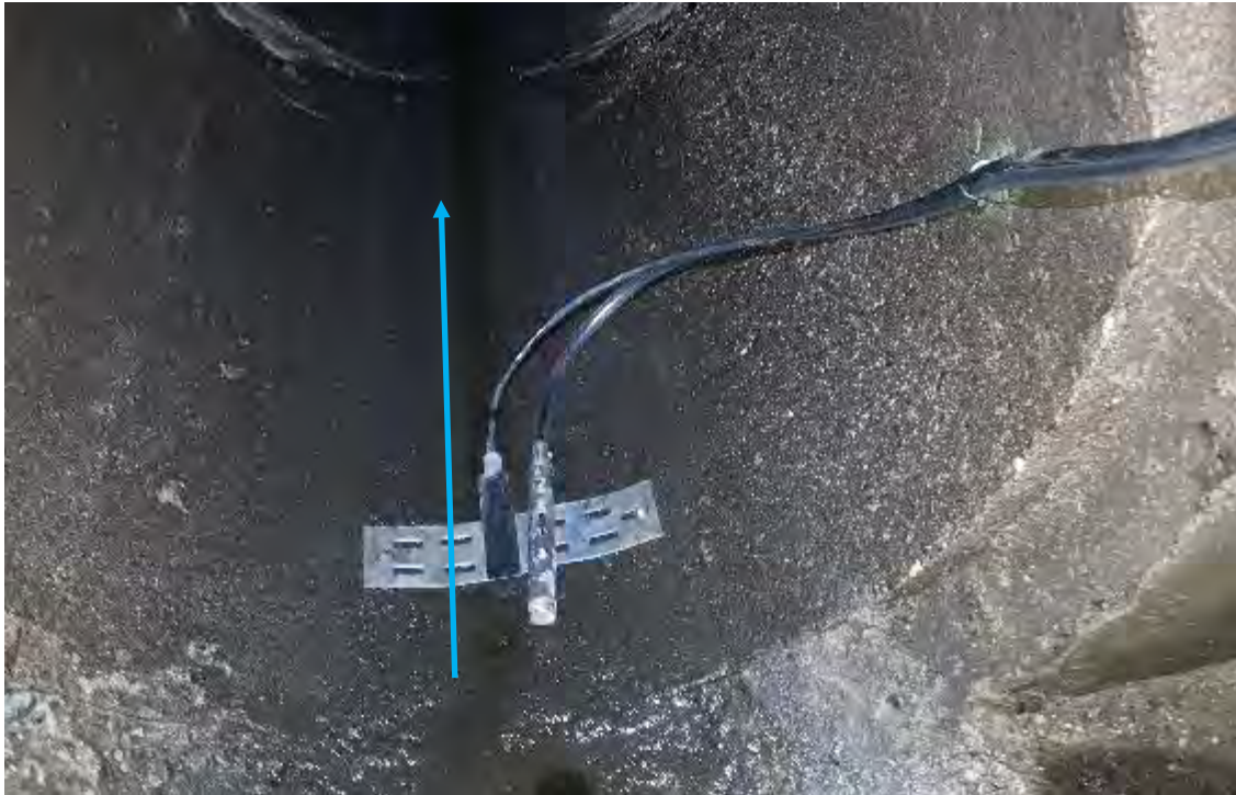
Figure 5. Photo of the AV probe and intake strainer at Powderhorn Inlet W in April of 2023. The equipment is attached to a stainless-steel plate that is bolted into the pipe. The blue arrow indicates the direction of water flow.
