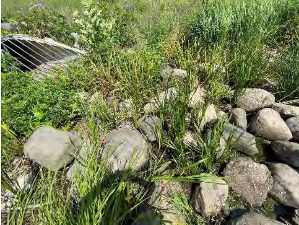
Figure 12. A photo of Camden Outlet taken on 7/11/23. The outlet structure can be seen on the upper left. Note the rip rap and the vegetation growing between boulders. Some pond water can be seen in the lower right corner.
