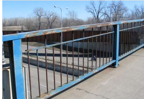
Corroded Guard Rail
