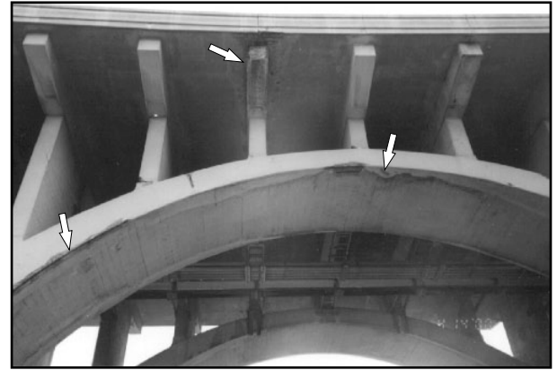
Arch and Floor Beam Deterioration
