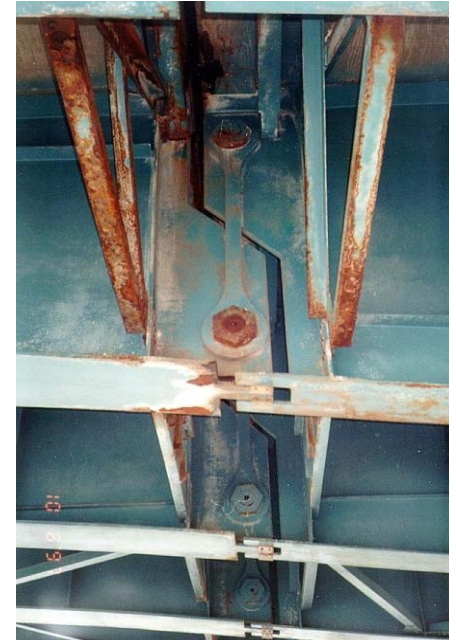
Corroded Pin Hinge & Bracing
