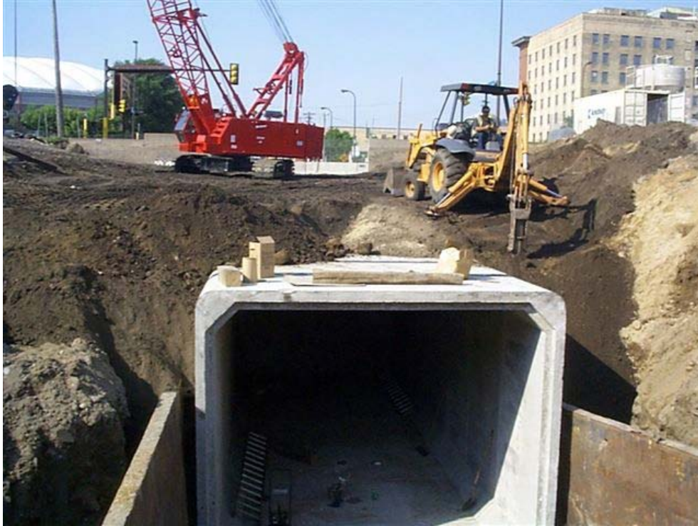
The Mill Quarter Regional Stormwater Facility
