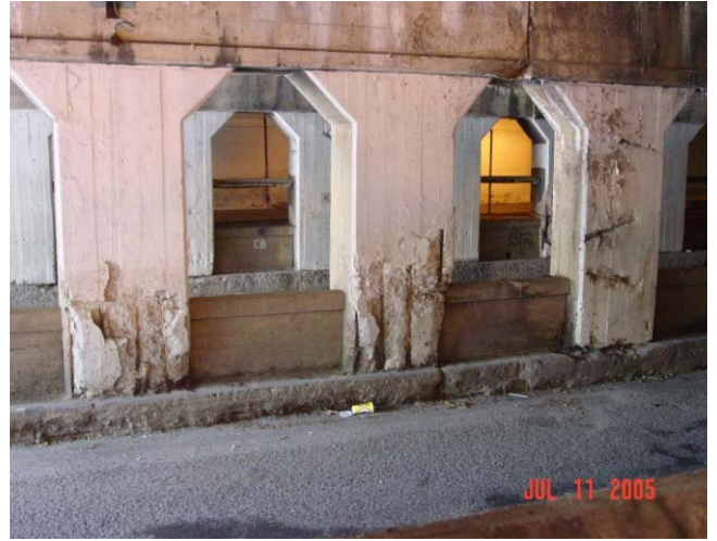
General Bridge Deterioration
