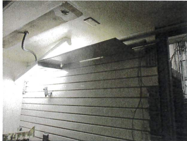
4-Foot Fluorescent Light – Utility Room
