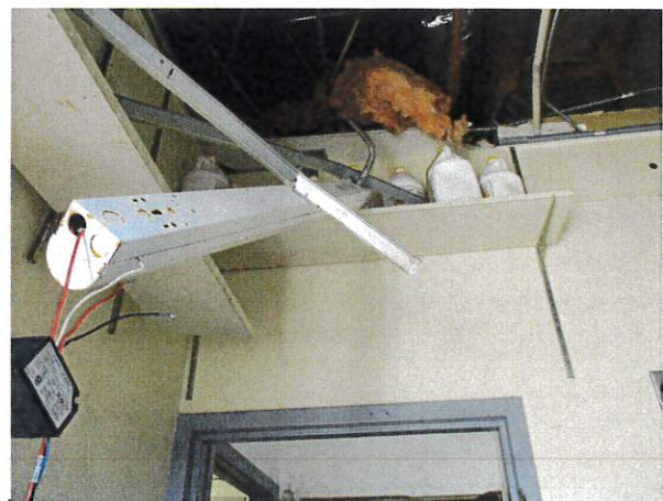
Fluorescent Light Ballast and Cleaning Solution – Janitor's Closet
