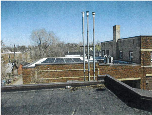
UST Vent Pipes –along the North Wall of the Former Gas Station Building
