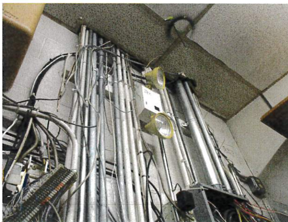
Security Lights – Utility Room
