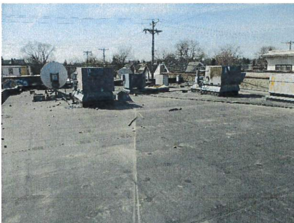
Central Air Conditioners and Satellite Dishes
