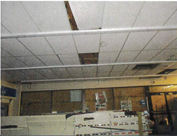
8-Foot Fluorescent Lights – Convenience Store
