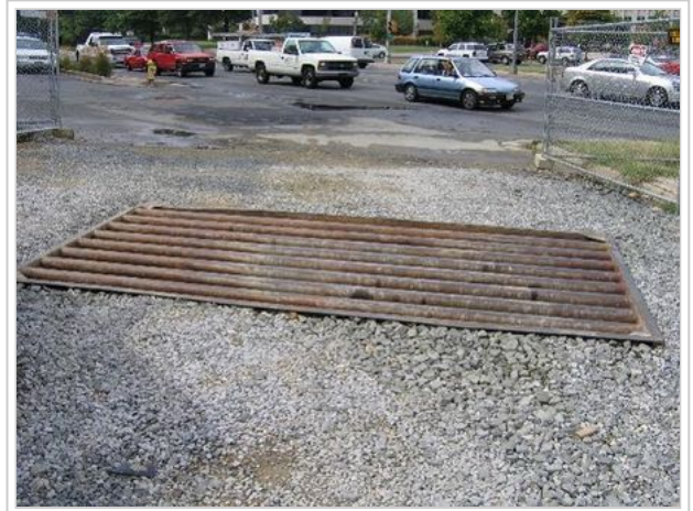
Example shaker rack installation. Source: Tetra Tech.
