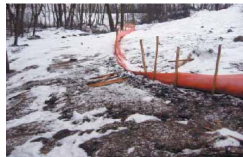
Regular maintenance is needed to ensure that a site's perimeter control is functioning properly.
