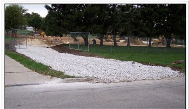
Example vehicle tracking pad. Source: City of Milwaukee.
