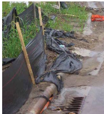
Planning ahead is the most effective way to minimize erosion and sedimentation during construction and reduce project costs.
