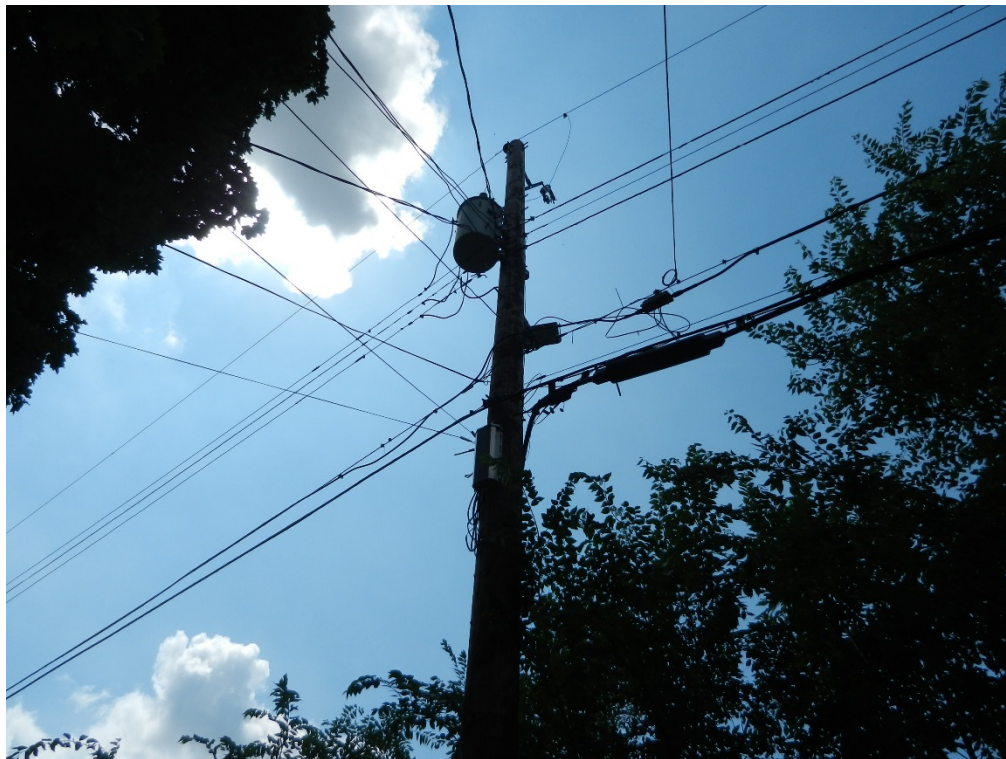
View of pole-mounted electrical transformer at 3206 Penn Ave N parcel
