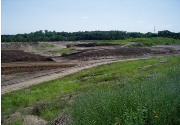
Leave as much vegetation on a site as possible to reduce the overall disturbed area.
