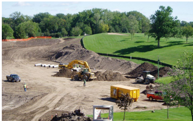
The NPDES permit requires that all erosion and sediment BMPs be clearly outlined in a site's SWPPP. Changes made throughout construction should be documented in the SWPPP.
