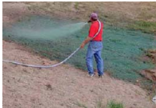
Hydrodraulic soil stabilizers promote the rapid growth of vegetation and prevent erosion.
