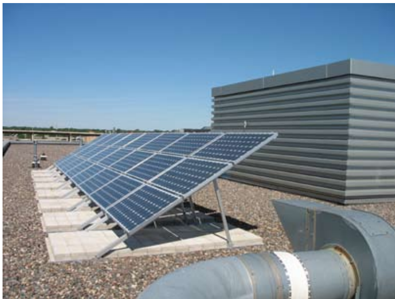
The Currie Maintenance Facility's solar array is one of three owned by the City of Minneapolis. The three photovoltaic systems produced 12,500 kWh of electricity last year.
